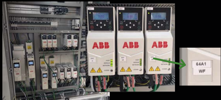
ON THE INVERTER DEDICATED TO THAT AXIS
